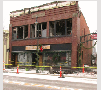
A Christmas Eve fire gutted the Cherry Republic building at 221 Bridge Street in downtown Charlevoix and left a number of nearby businesses with smoke damage. It was the second fire to destroy a business within a two block stretch of Bridge Street in the last two months.
